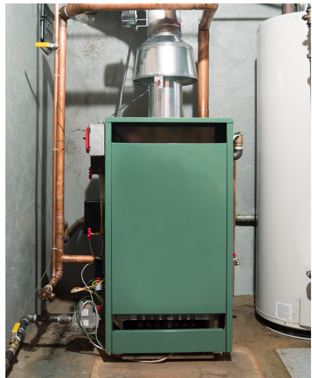
A typical hot-water boiler
